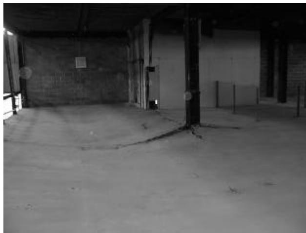
Figure 3 - Typical Post-Fire Damage to Composite Slab
