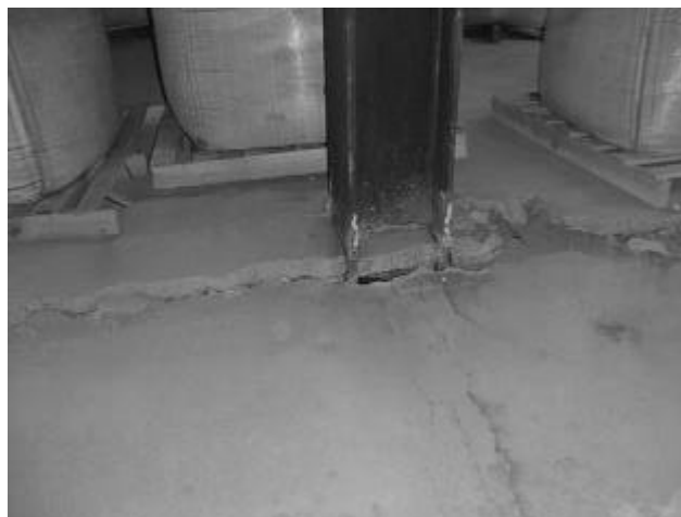
Figure 4 - Typical Post-Fire Damage to Slab at Column Perimeter in Composite Frame
