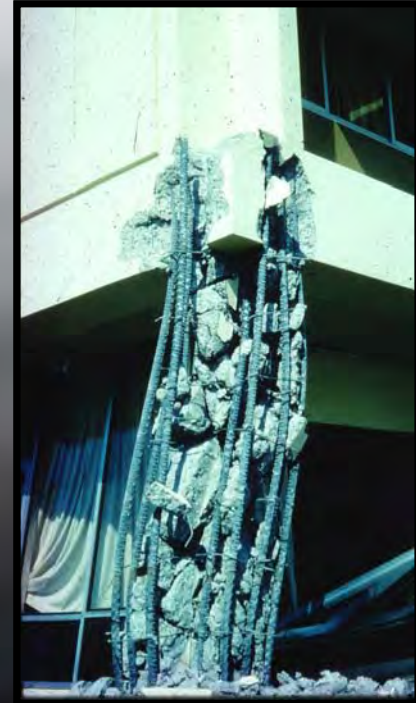
Poorly confined column Kobe, Japan 1995
