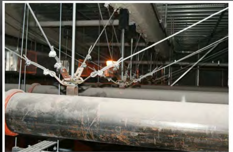
Figure 6.4.3.1-6 All-directional cable bracing of suspended piping (Photo courtesy of ISAT).
