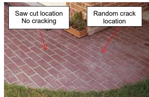
Figure 15 Cracking due to late saw cutting
