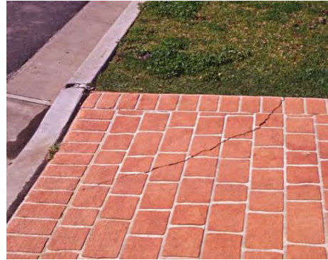
Figure 5 Ensure the ground is free of softer areas that may cause future cracking
