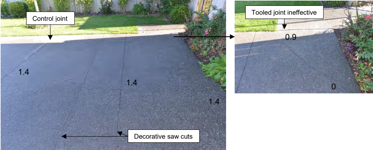
Figure 2 Example of cracking to driveway
