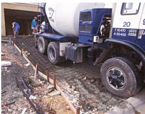
Figure 4 Inadequate lapping of mesh at corner
