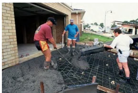
Figure 5 Inadequate lapping of mesh at corner
