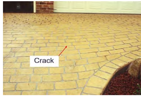
Figure 11 Cracking due to excessive joint spacing
