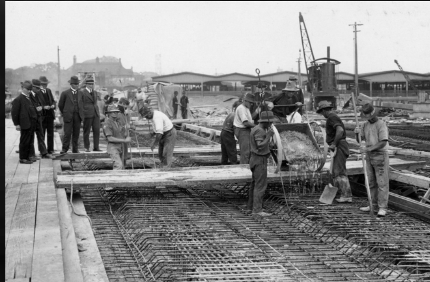
Concrete placement' 2 April, 1925 (Australian Railway Historical Society image 517470) Note: John Job Crew Bradfield CMG on left side of image inspecting the works.
