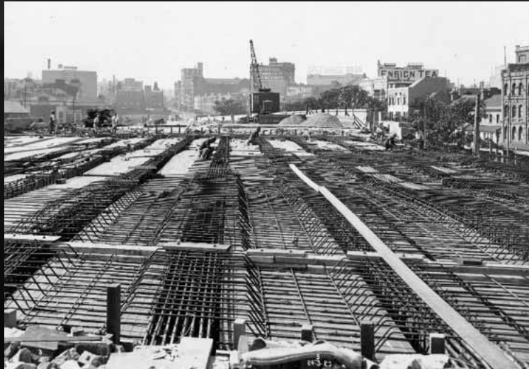
Railway bridge over Eddy Avenue on 24 March, 1925 (Australian Railway Historical Society image 517458)
