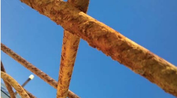
(a) Corroded mesh
