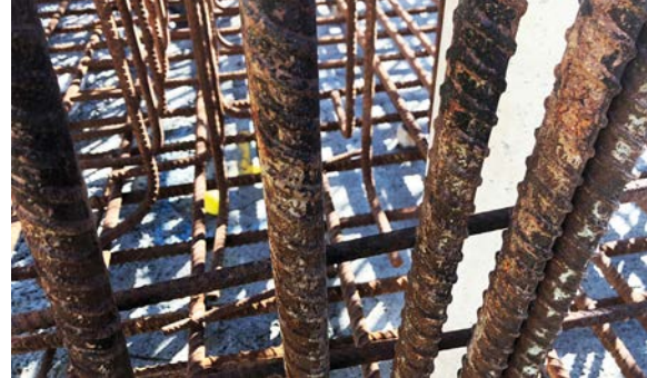
(b) Corroded column starter bars
