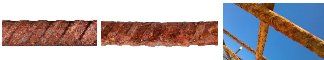
Figure 8 Examples of loose and flaking rust indicating loss of steel section
