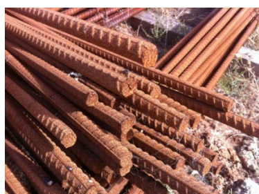
Figure 9 Example of acceptable surface corrosion
