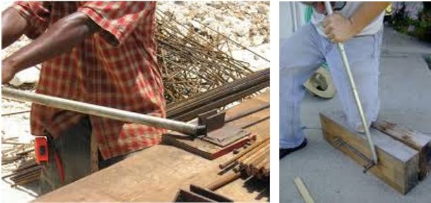
Figure 11 Common, but poor site bending practices no longer permitted in AS 3600
