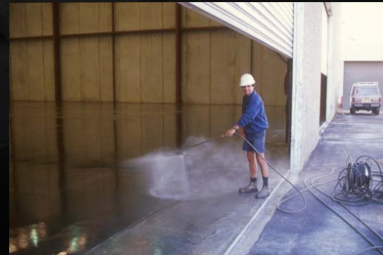
Retain water in concrete
