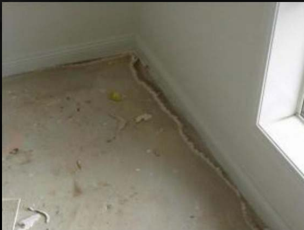
(courtesy New Home Inspections, Melbourne)
